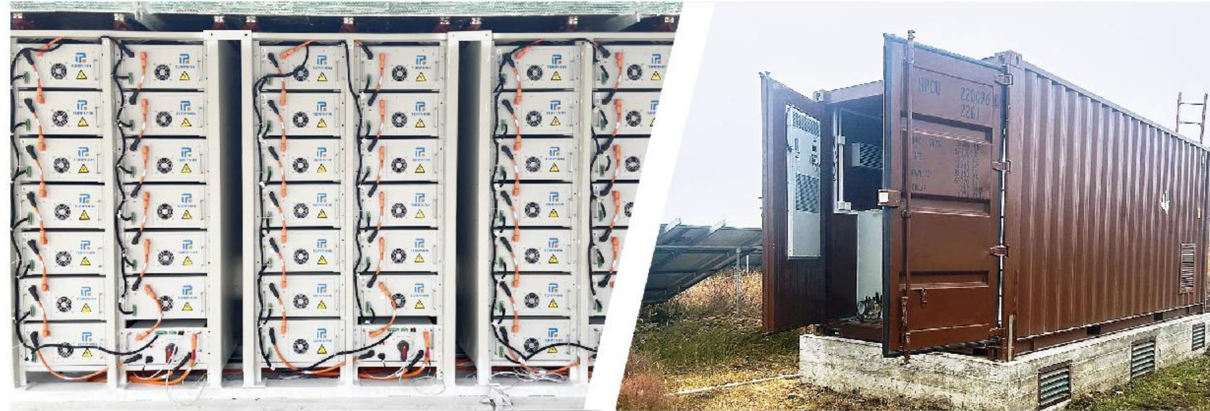
• Container Energy Storage System •
